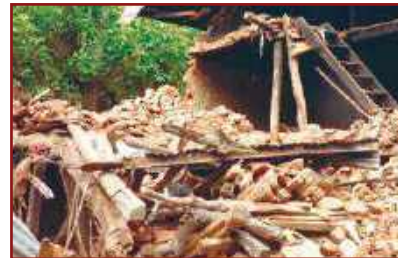
Falling debris from the upper storey or attic causing damage.
