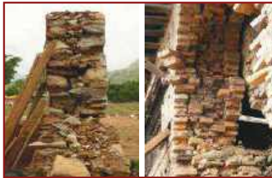
Faces of Stone and brick walls separate when Headers are not provided or are not enough
