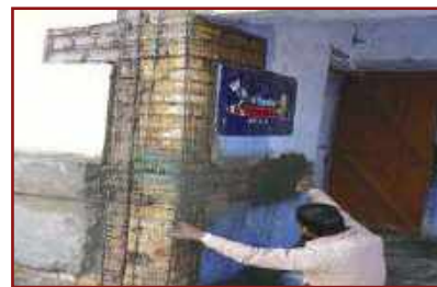
Full height wall to wall separation being rectified with WWM corner splint and additional straps.
