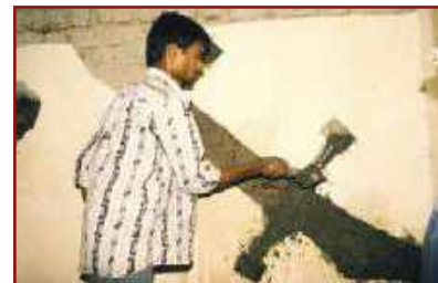
Plaster over the clamp and crack with two 12mm coats of 1:3 cement plaster.
