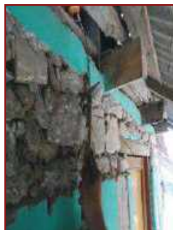
8. Chips must be hammered in strongly to ensure that they lock the stones around them.
