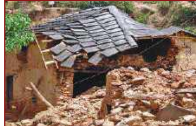
Collapsed roof due to collapsed walls
