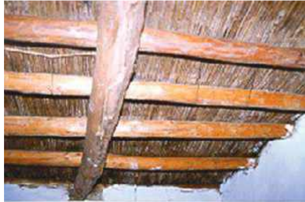
R.4.2 Inadequate and poor floor members
