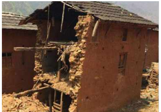
Figure 4: Collapsed gable wall
