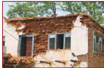
Delamination of a thick brick wall
