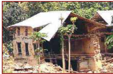
Damaged roof because of severe damage to the support walls and other support systems.
