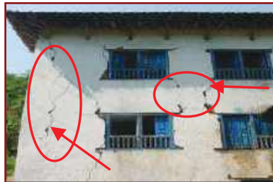
Grade 3 cracks in plastered wall
