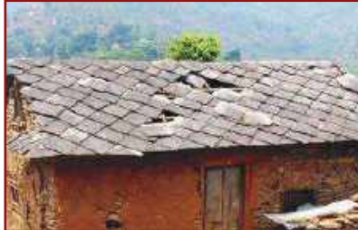
Damaged roof structure and dislodged slate / roof tiles
