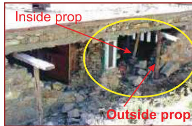
Props placed inside as well as outside the building to support the slab
