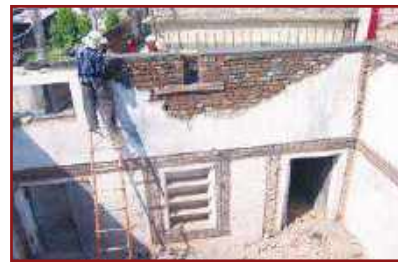
Damaged brick masonry wall being rebuilt to reinstall RC slab on it.
