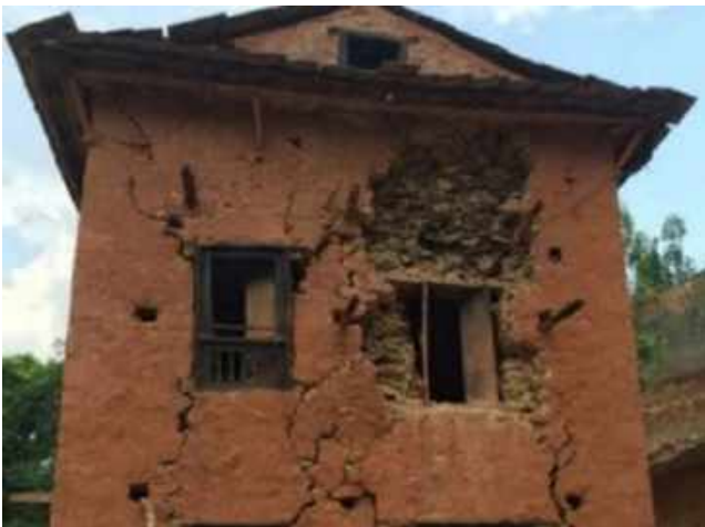
Figure 3: Short wall out-of-plane damage in SMM building
