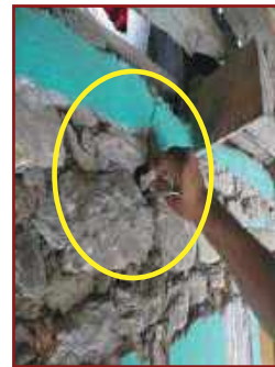
7. Insert small stones or stone chips below and above the cross links using little mud mortar for closing the hole.
