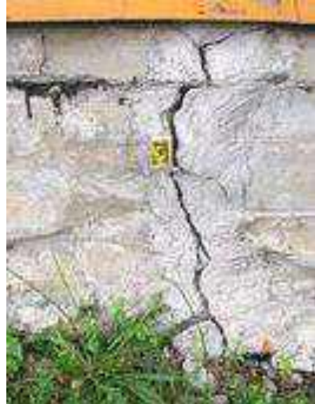
F.2 Settlement of Foundation
