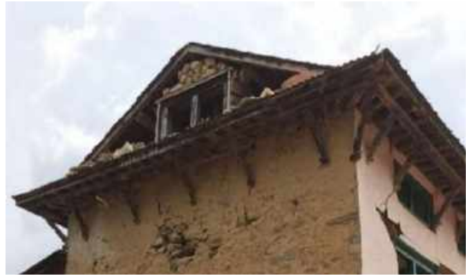
Figure 2: Damaged gable wall in an SMM house
