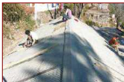
Nails being replaced by 'J' hooks to anchor tin sheets to purlins.
