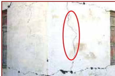
Grade 2 cracks in wall with Cement plaster.
