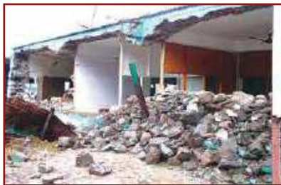
Undamaged RC slab on severely damaged wall
