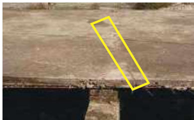
Grade1/Grade 2 Crack in RC roof/floor
