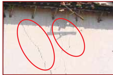
Grade 2 cracks in Cement plastered wall
