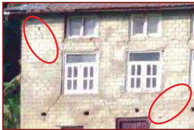
Exposed masonry wall having Grade 2 cracks
