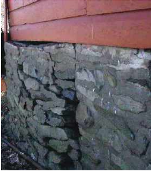
F.3 Bulged and leaning stone Foundation
