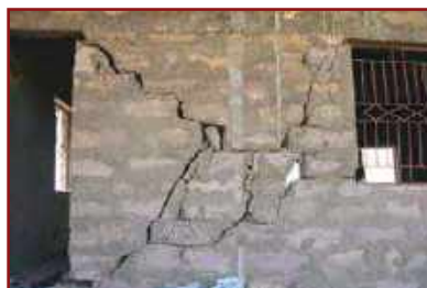
Grade 3 cracks between opening
