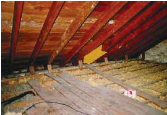
R.4.1 view inside the attic showing the rafters and the absence of collar beams and joist connections to the rafters
