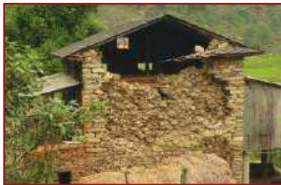
Separation of a face followed by delamination of part of a stone wall
