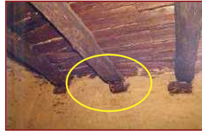
Sliding of timber joists sitting on bearing stones projecting out from walls.
