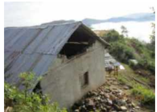
Figure 5: Attic wall out-of-plane damage (Photo credit: NRA)
