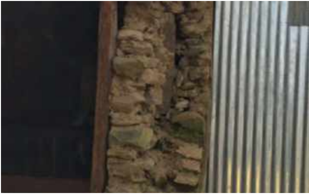
Figure 1: Cross section of a damaged SMM house showing the dual layer of stones
