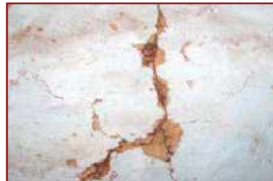
Grade 2 cracks in wall with mud plaster
