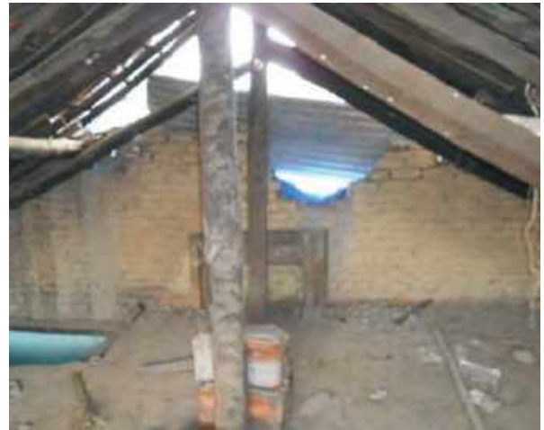
R.1.2 Gable wall toppling
