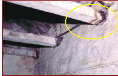
Sliding out of timber joists sitting on walls
