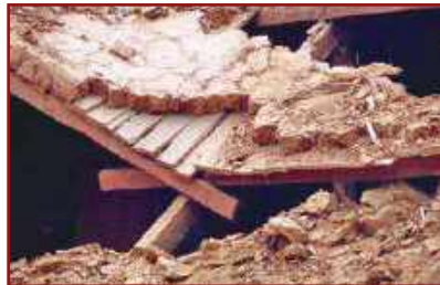
Breaking of floor joists
