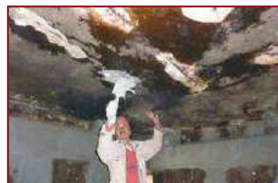
Spalled concrete removed, rusted bars cleaned and coated with anti-rust chemical, bonding agent applied and finished with micro-concrete.
