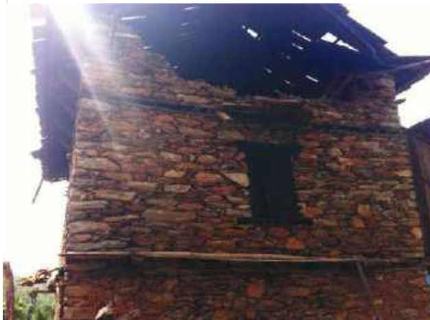
R1.1 Gable wall toppling
