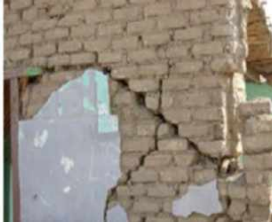
Figure 7: In-plane damage in wall
