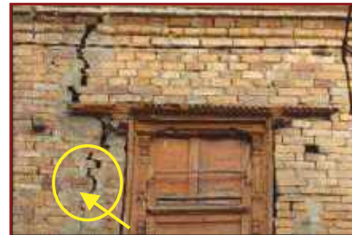
Grade 3 cracks in un-plastered wall
