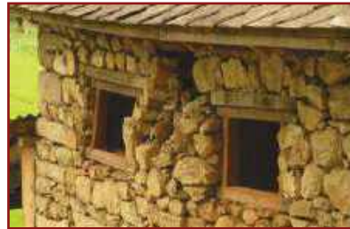
Bulging of outer face of thick stone wall
