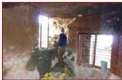
Badly damaged stone masonry wall dismantled and being rebuilt accompanied by a new window.
