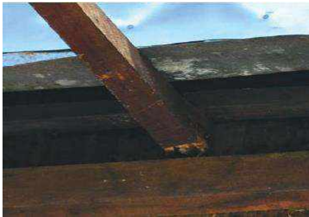
R.3.1 Purlin detached from rafter due to inadequate nailing
