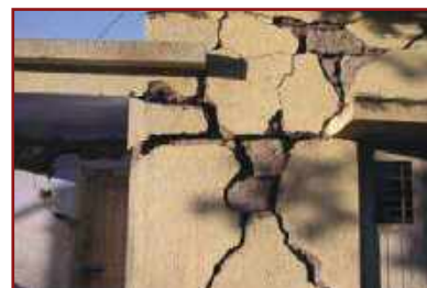
Grade 3 cracks in masonry
